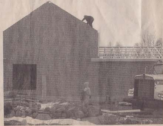
Workers from Terry's Barn Restoration of Three Rivers assemble parts of an old barn in their effort to help Southern Exposure rebuild.
